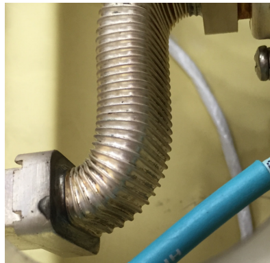
Figure 5 Excessive Bending of the Flex Section
